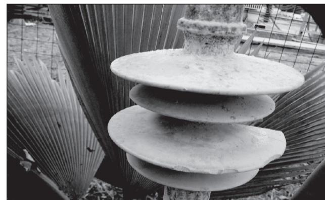
PH. 5 SCALE FORMATION ON SRV INSULATOR
