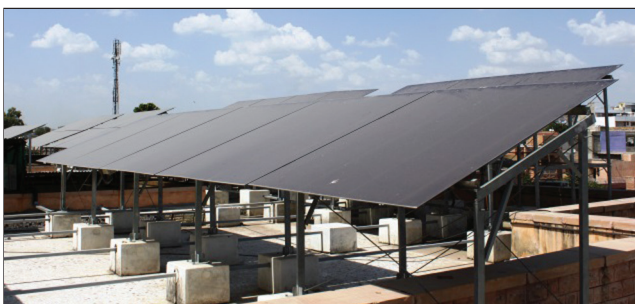
FIG. 5 A-Si BASED 43 kW ROOFTOP GRID TIED SOLAR PHOTO VOLTAIC SYSTEM
