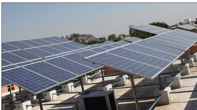
FIG. 2 C-Si BASED 58 kW ROOFTOP GRID TIED SOLAR PHOTO VOLTAIC SYSTEM.
