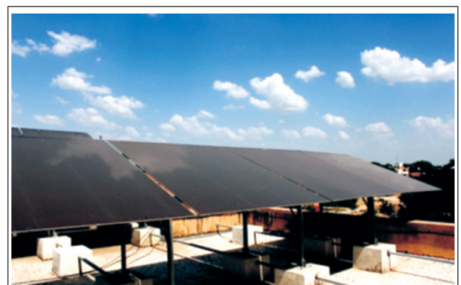
FIG. 3 A-SI BASED 43 KW ROOFTOP GRID TIED SOLAR PHOTO VOLTAIC SYSTEM
