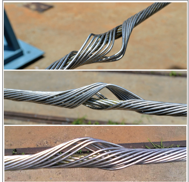
FIG. 8 BIRD CAGING OF OPGW DUE TO SHORT CIRCUIT CURRENT
