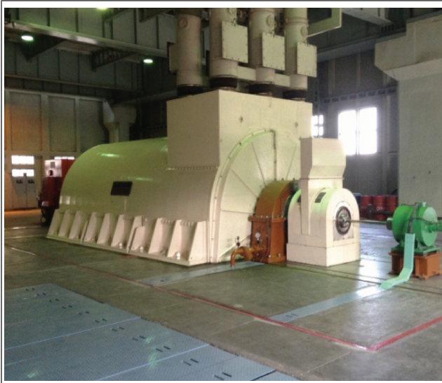
FIG. 1 A VIEW OF SHORT-CIRCUIT GENERATOR AT CPRI, HIGH POWER LABORATORY, BANGALORE
