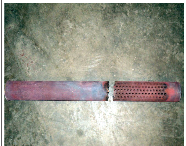
FIG. 5 IMAGE OF BROKEN INJECTOR TAKEN OUT FROM ATTEMPERATOR
