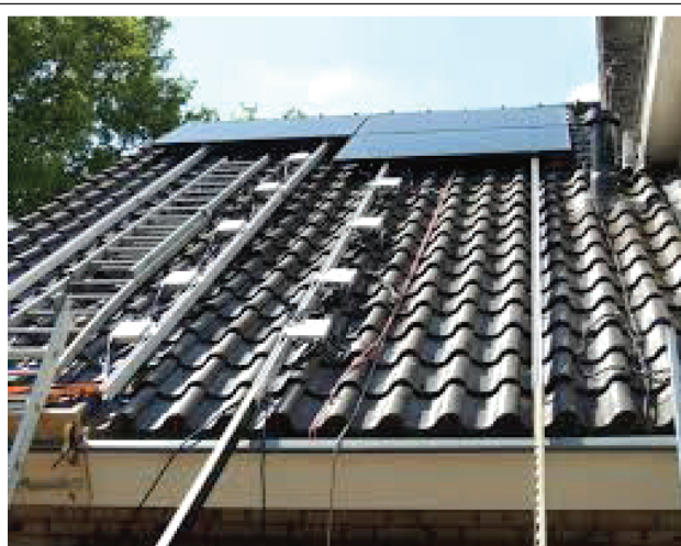
FIG. 5 ROOF TOP MICRO INVERTER
