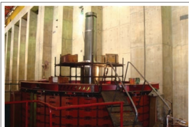
FIG. 1. VIEW OF GENERATOR SHAFT WITH ROTATING MASS
