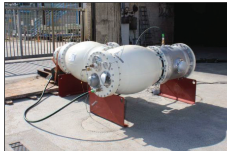
Figure 7. Test setup for clean air GIS [Courtesy Siemens Energy] (before test).
