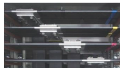
Figure 11. Sleeved busbars with > 25mm clearance.
