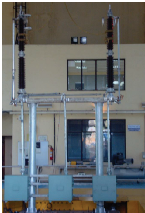
Figure 7. 245 kv horizontal centre break disconnector: Disconnector open and ground switch closed.
