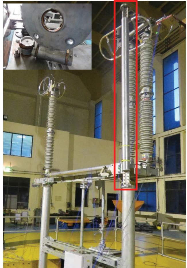
Figure 6. 245 kv disconnector main contact tube dislocated.
