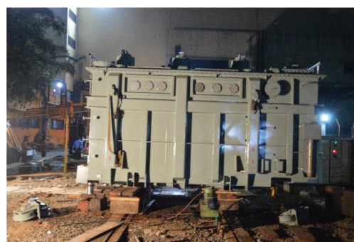
Figure 4. Testing of 50 MVA, 110/22/11 kV, 3 winding oil type transformer insulation at 100KV switchyard.
