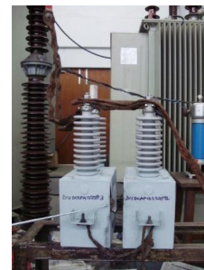
Figure 2. A view of two capacitors connected in parallel-undergoing OVC test.
