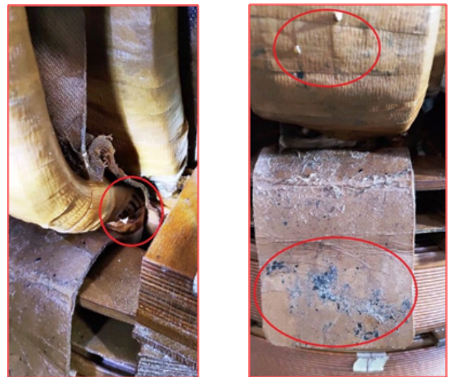
Figure 11. Photographs of the fault in Y phase LV winding with insulation puncture and carbon particles due to discharge.
