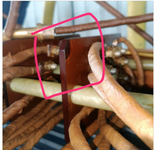
Figure 21. Photograph of the fault in B phase winding.
