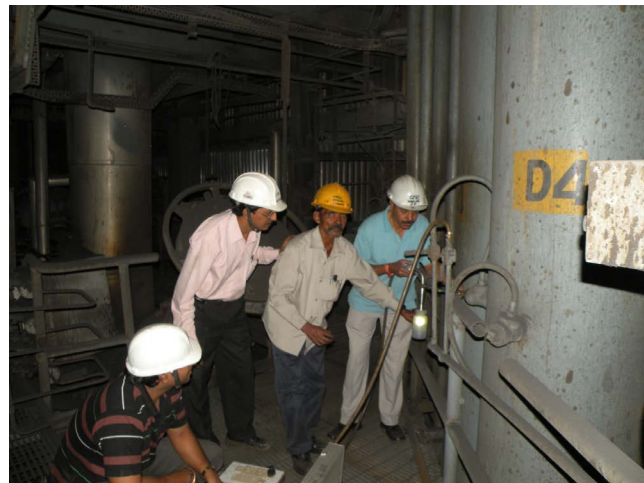
Figure 3. ISO kinetic coal sampling from coal duct.
