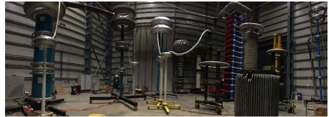
Figure 11. Example of a Test set-up for the slow impulse type dynamic voltage test.
