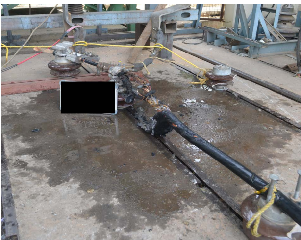
Figure 3. Thermal failure in HT cable
