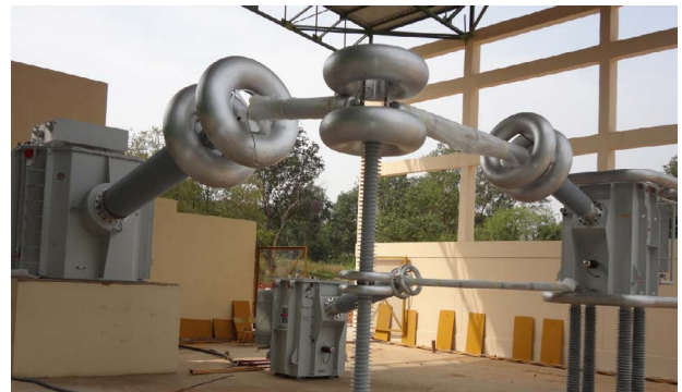
Figure 1. 600 kV, 4200 KVA transformer.
