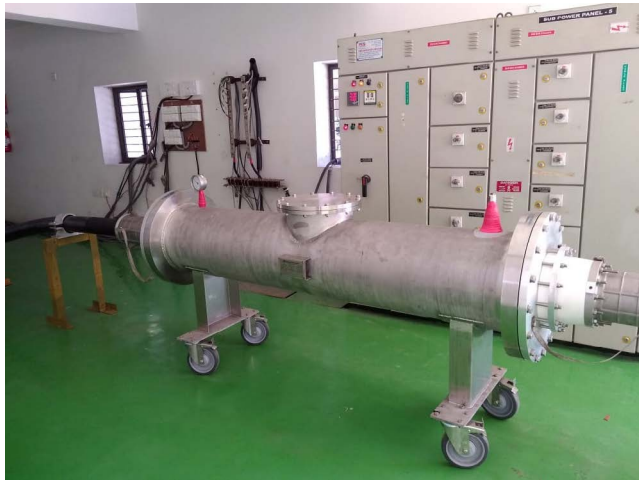
Figure 5. SF6 back to back joint.
