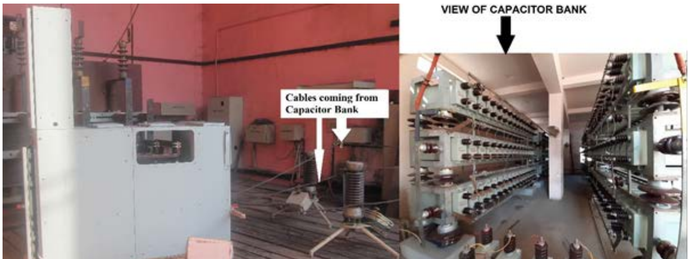
Figure 4. Testing sample arrangement during Capacitor Switching of 12kV, 26.3kA Indoor VCB with Panel.
